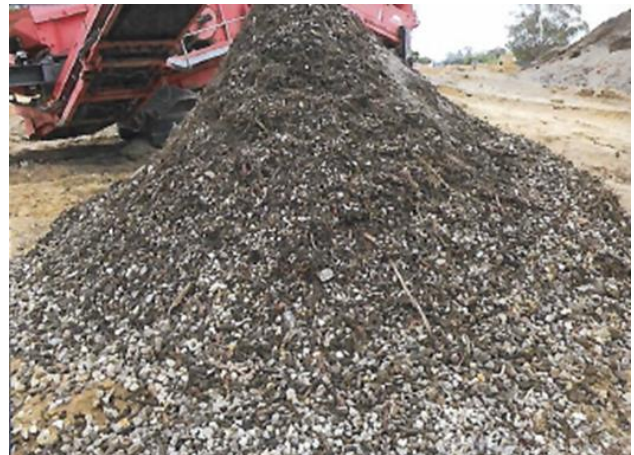
Topsoil screening for direct on-site reuse at The Amble Estate. (Image supplied by Porter Consulting Engineers)
