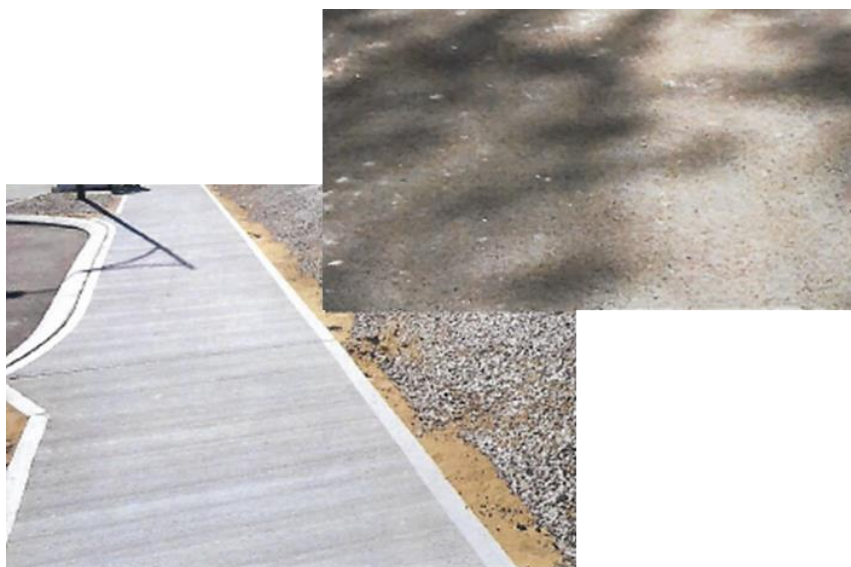
Path and pavement incorporated recycled product – concrete, sand, and asphalt. The Amble Estate (Images supplied by Porter Consulting Engineers)
